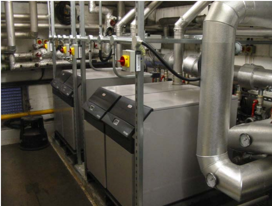
Photo 6: Boiler room with well lagged pipes
