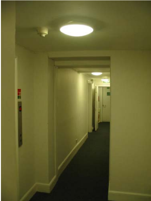
Photo 5: Excessive lighting in corridors
